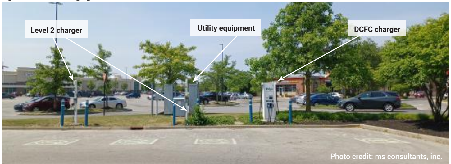
Figure 0.1 An EV charging station
